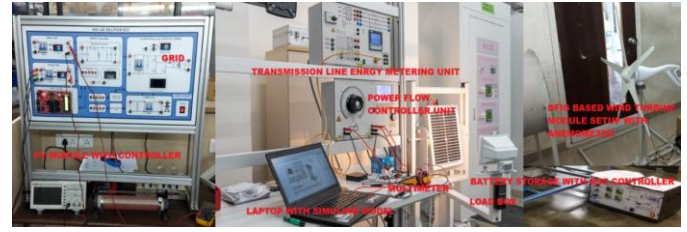
Fig. 8. Hardware setup of PV-Wind-BESS model with energy meter unit.
